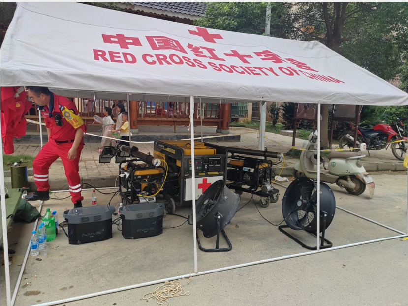
Temporary Emergency Power Supply Station in Disaster Area
